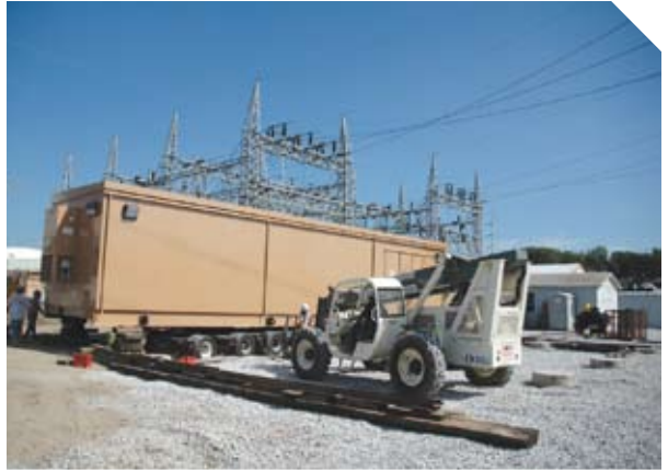
ELECTRICAL SUBSTATION PROJECT IN RALSTON, NE
