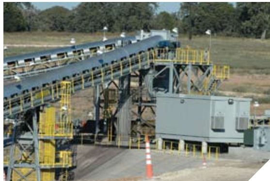
ELECTRICAL EQUIPMENT CENTER AT AGGREGATE MINING FACILITY
